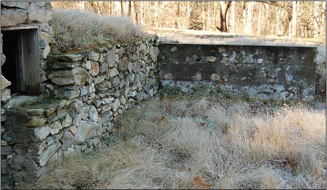
Figure 15. Looking west along west barn shed foundation wall, at left, showing where it abuts west silo and concrete foundation wall
