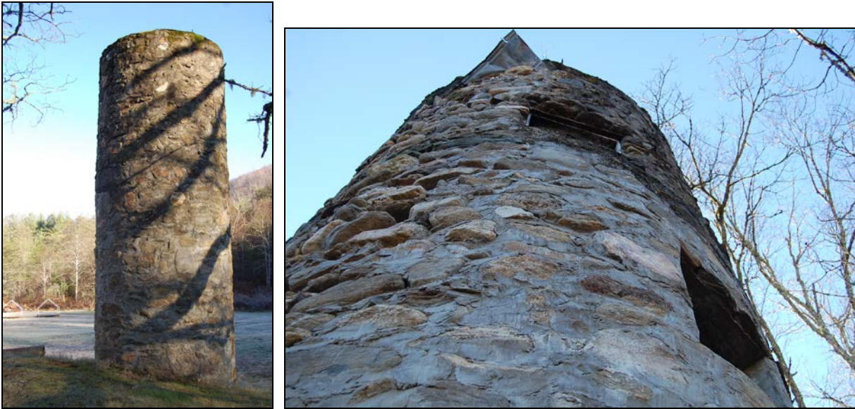
Figure 24. East Silo: south face at left; west/northwest face at right with re-mortaring evident, original uppermost opening at top center, and piece of barn roof sandwiched into stonework near the top
