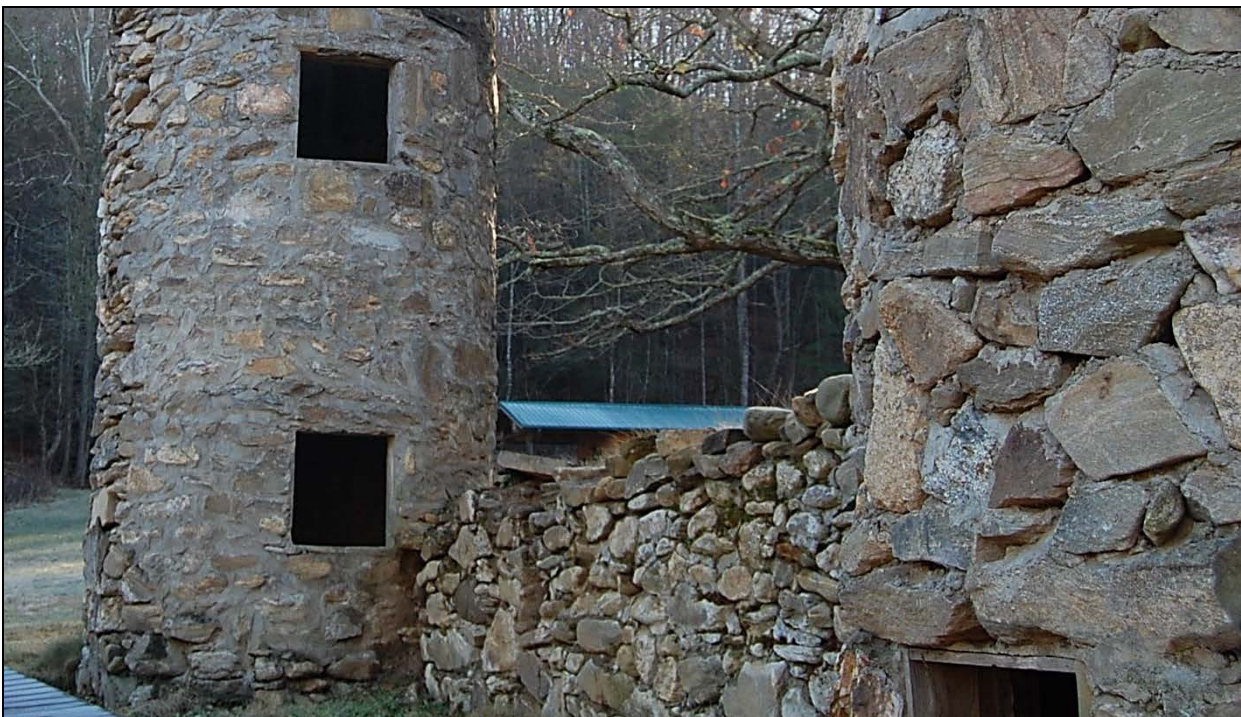
Figure 18. Looking southeast along length of south shed foundation wall between west silo, at right, and east silo, at left
